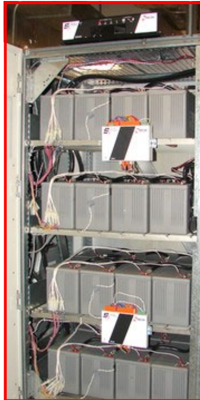
VRLA battery string
